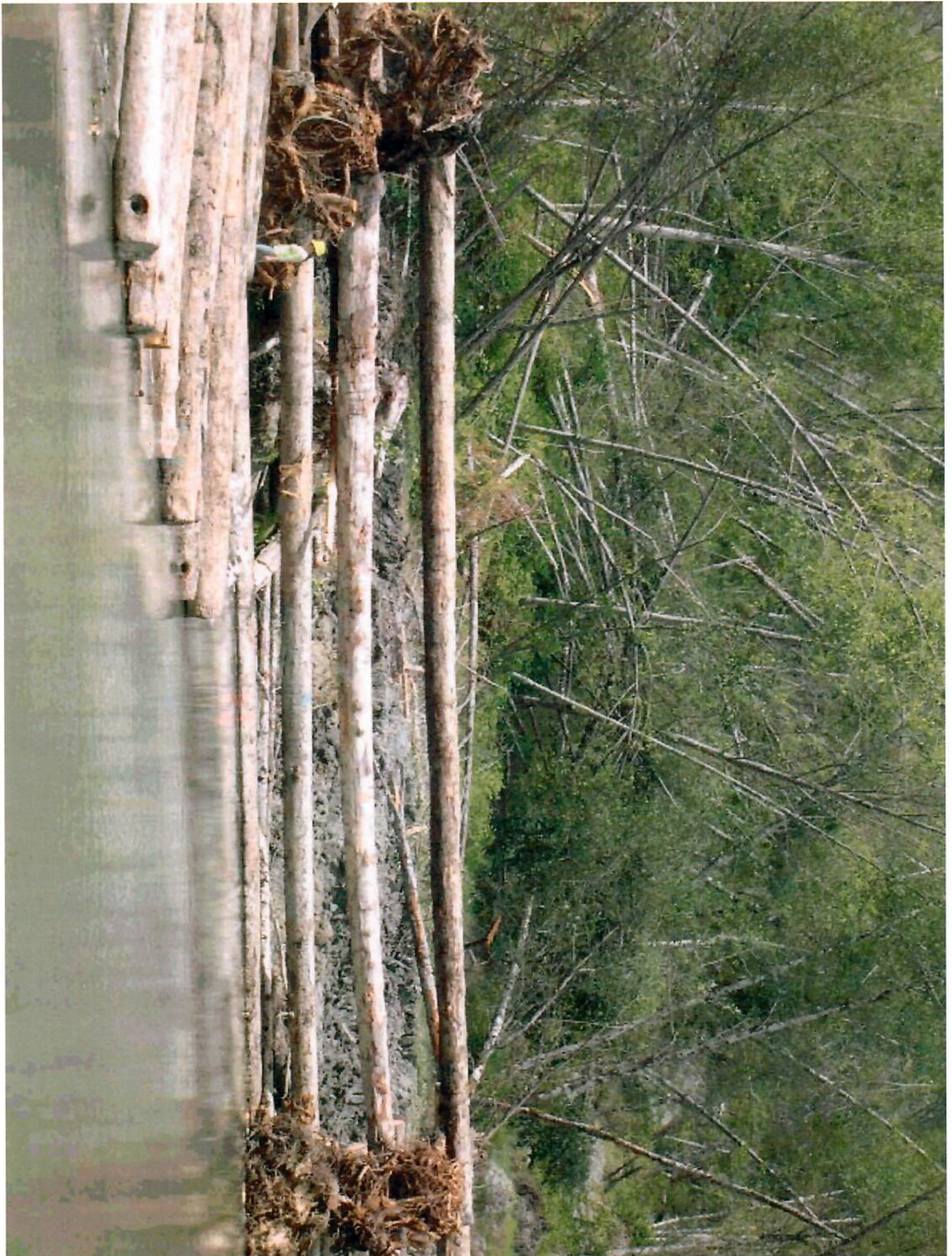
Close-up look at log jam revetment. Notice person on left for scale.
